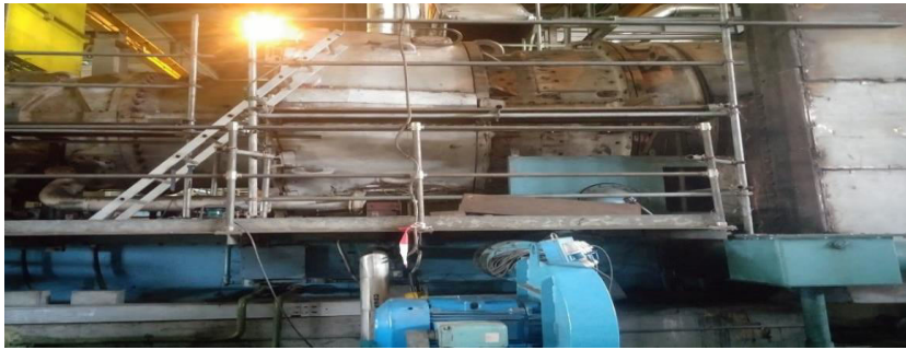
Figure 5: General Electric (GE) Frame 9E Gas Turbine Prepared for Combustion Inspection at TPL
