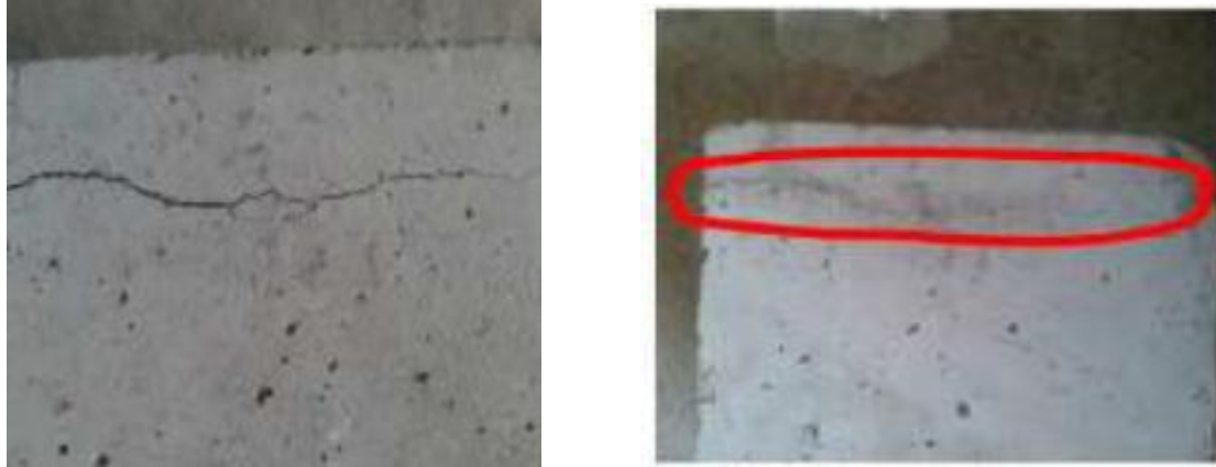
Figure 4: Cube with initiated crack b) Healing of crack due to B. Subtilis by M.I.C.P
